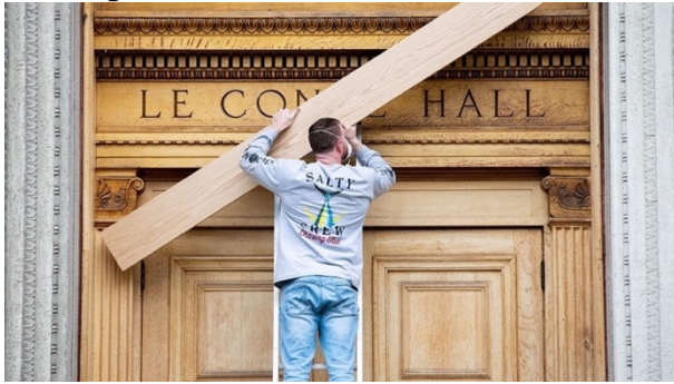
Figure 20. UC Berkeley employee using plywood to cover the words “Le Conte Hall” inscribed at the entrance of the building now named Physics South.
